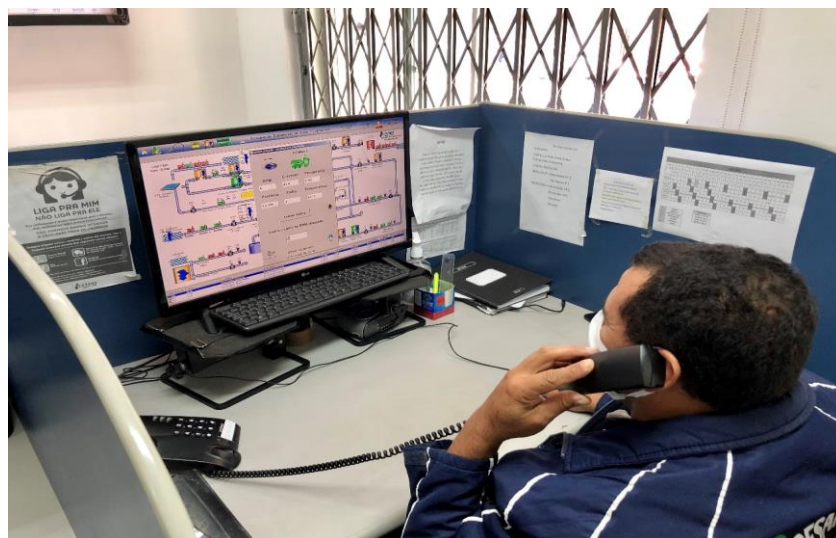
Cesama's Operational Control Center
