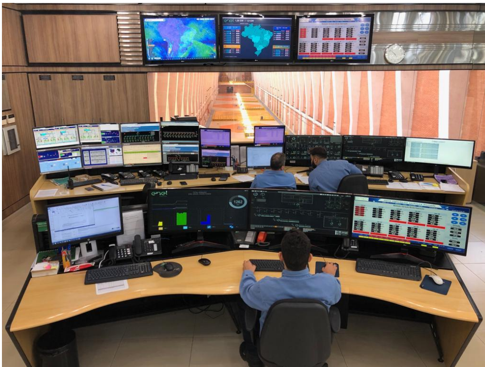
Enel's Generation Operations Center (GOC)
