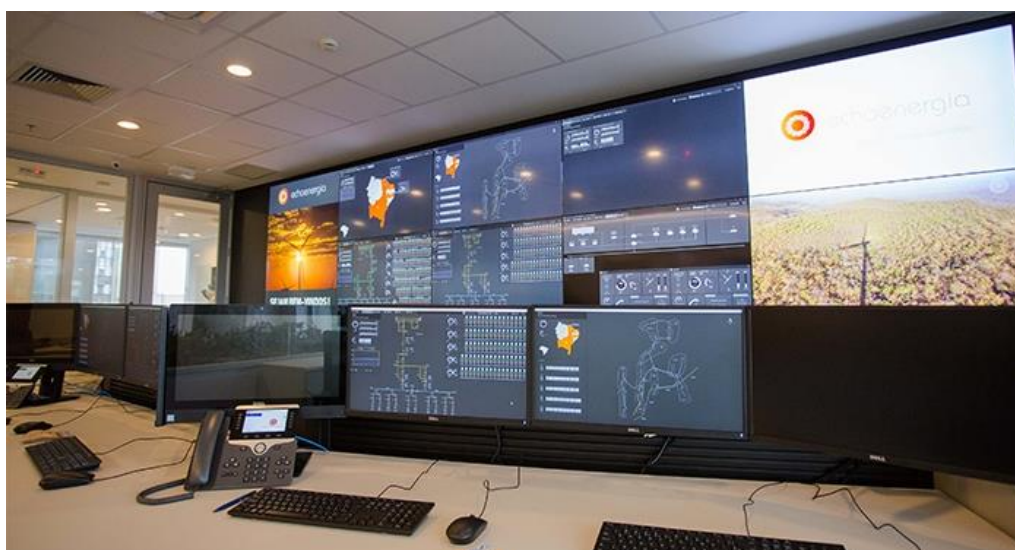
Figure 1. Echoenergia's Generation Operations Center
